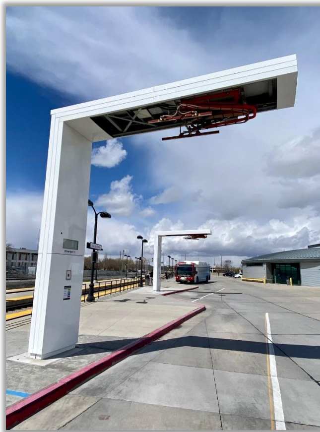
Figure 4. Overhead Chargers at the Salt Lake Central Station.
