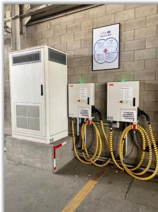
Figure 3. Plug-in Charging Infrastructure at Central Business Unit
